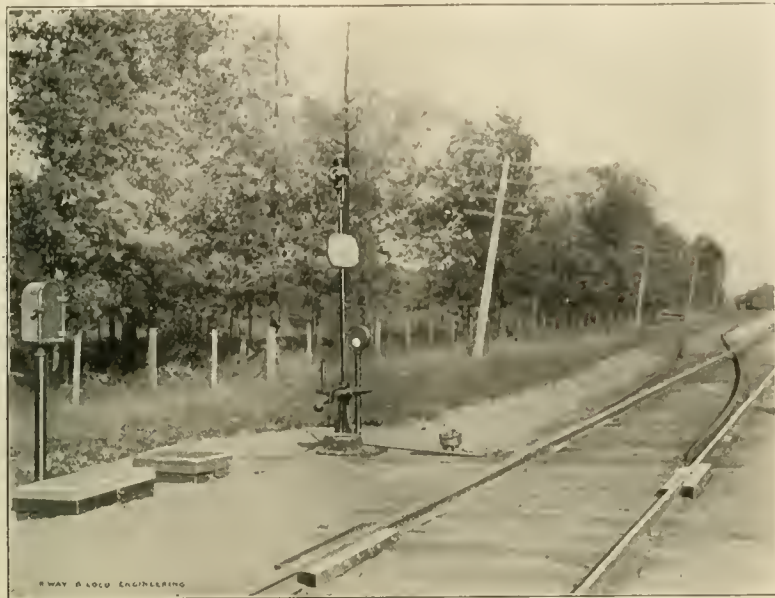
SWITCH STAND AND TARGET WITH SWITCH INDICATOR BESIDE IT. TRACK INSULATION SHOWN AT END OF BLOCK.
